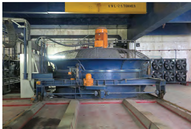
A massive 1960s automated fan, pulling clean fresh air into the tunnel, coming up through the tunnel kerbstones.
